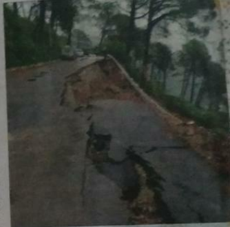
The damaged Dharamsala-McLeodganj road. PHOTO: ANIL MEHTA
