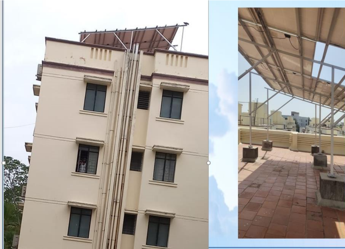
Fig.7. Micro Solar panel installed in a housing colony
