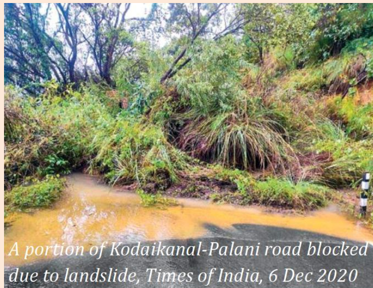
Fig.2d(viii): Damages due to CS BUREVI
