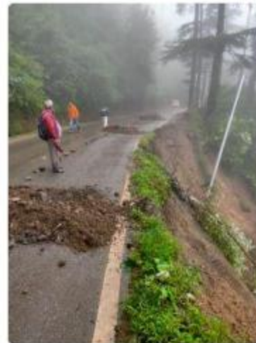
Road damage at Rd 14/00-14/030 on NH 05 at mahali road single lane due to damage of outer road edge due to sliding
