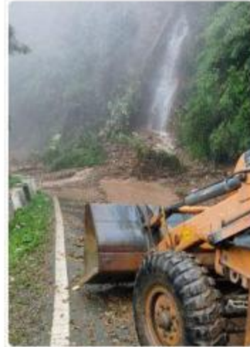
Shimla Airport road blocked at various RD Machinery deployed for removal of slips
